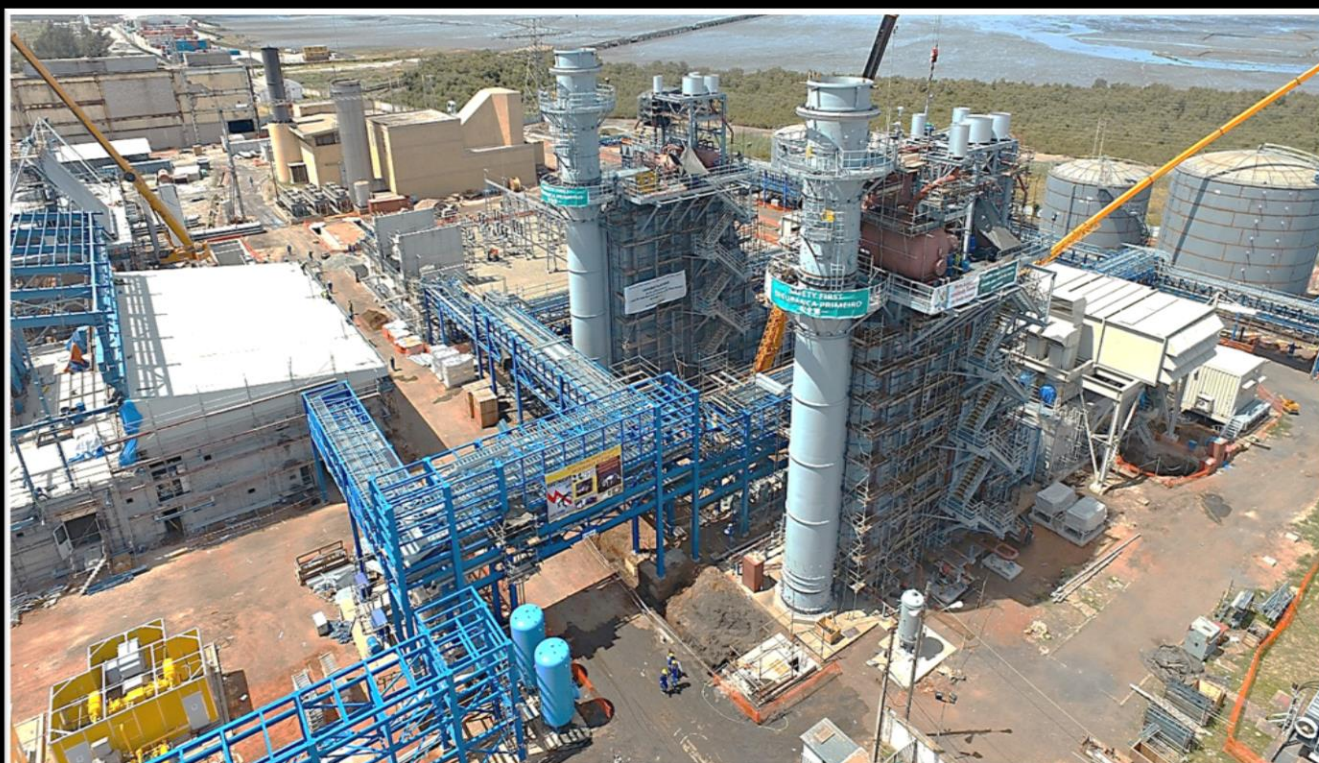
Maputo Gas Fired Combined Cycle Power Plant Development Project site
