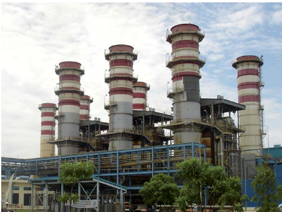
Partial view of the existing Muara Tawar gas-fired combined cycle power plant.
